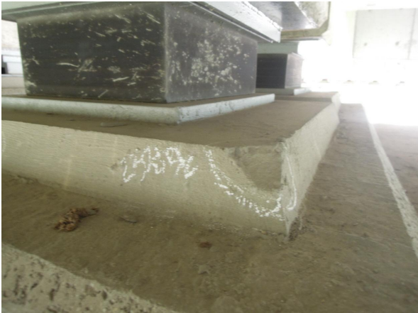
교각 P2-SH6 받침몰탈파손(0.1m×0.1m)
