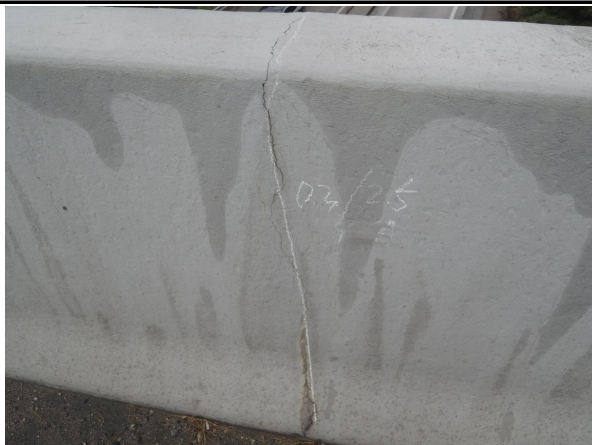
S1 방호벽 균열(0.3mm/2.5m)
